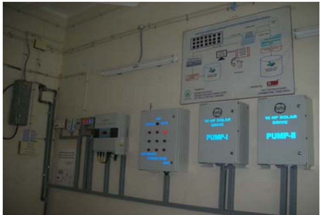
Fig. 4 10KW PV solar and pump control room
