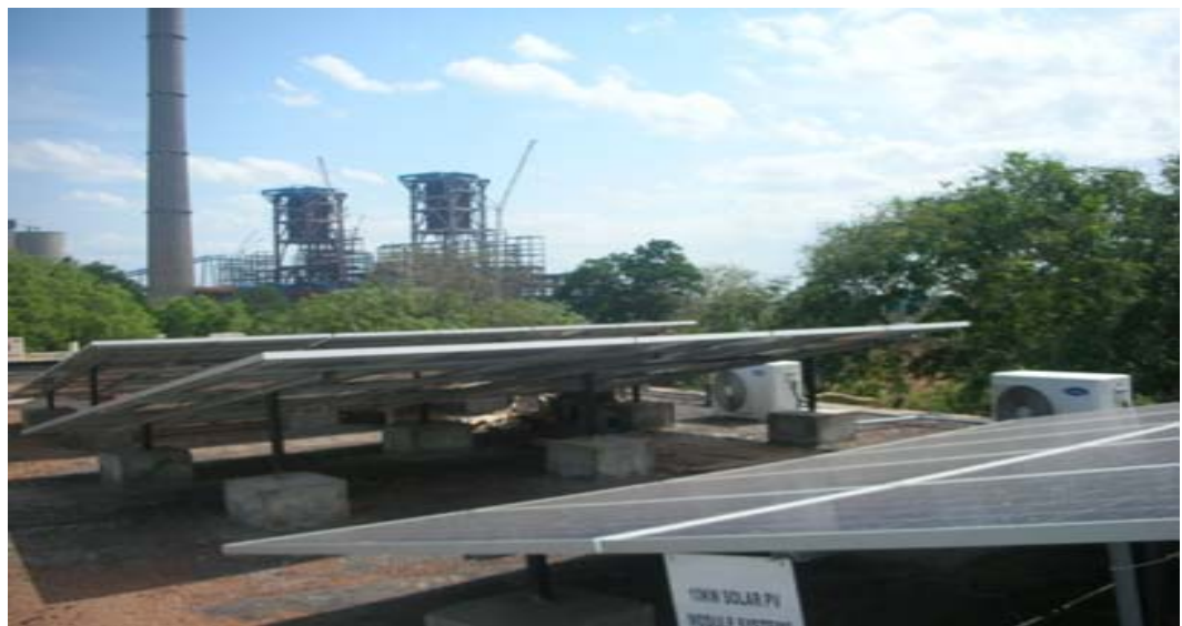
Fig. 2 10kw Roof top solar PV panel mounting
